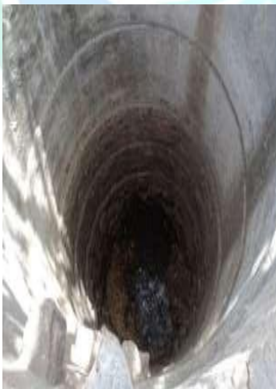
Dry open well in June
